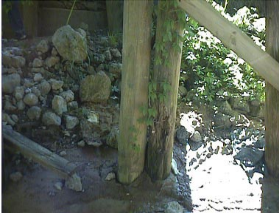
TIMBER BRIDGE PILE WITH DECAY
