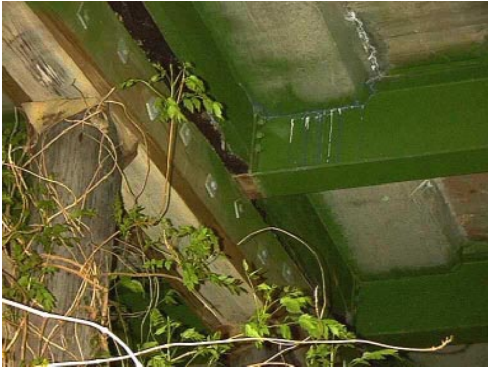
CAPBEAM MOVEMENT AT BENT #8
