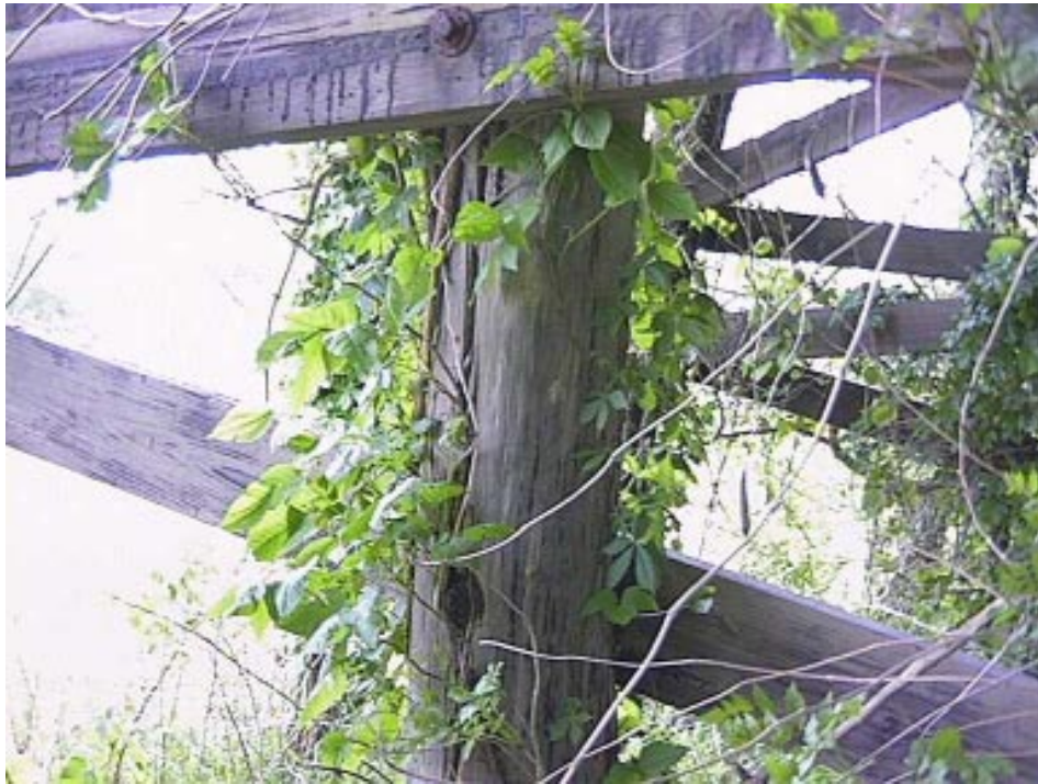
SEVERE DECAY IN INTERIOR TIMBER PILE "B"
