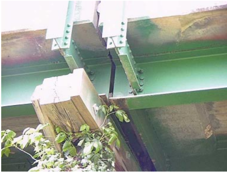
LOSS OF BEARING ON CAPBEAM - EXTERIOR BEAM "A"
