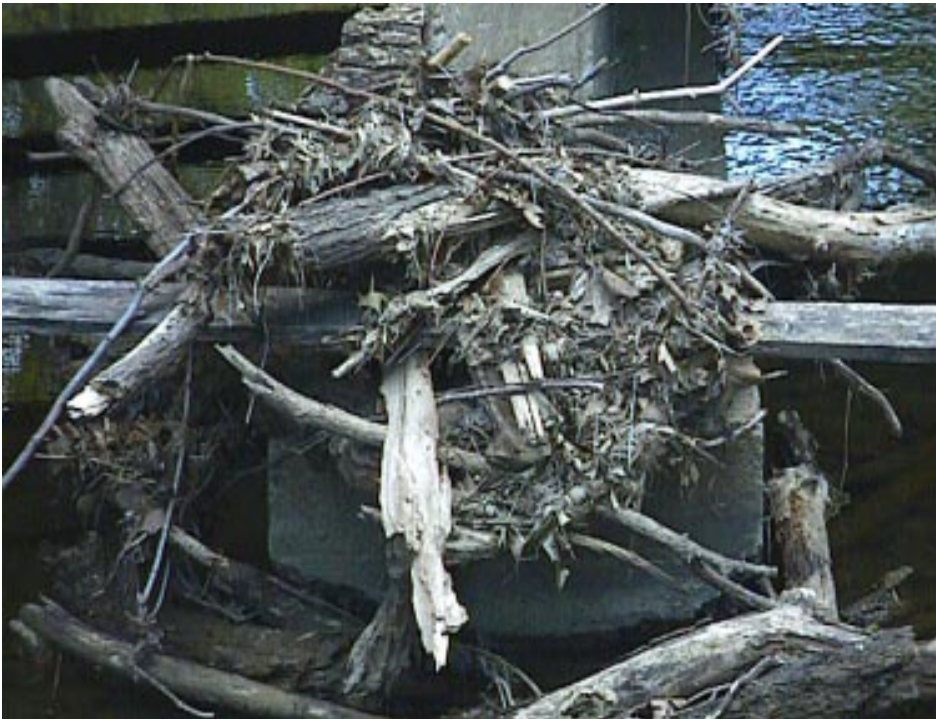
DRIFT AT BRIDGE PIER
