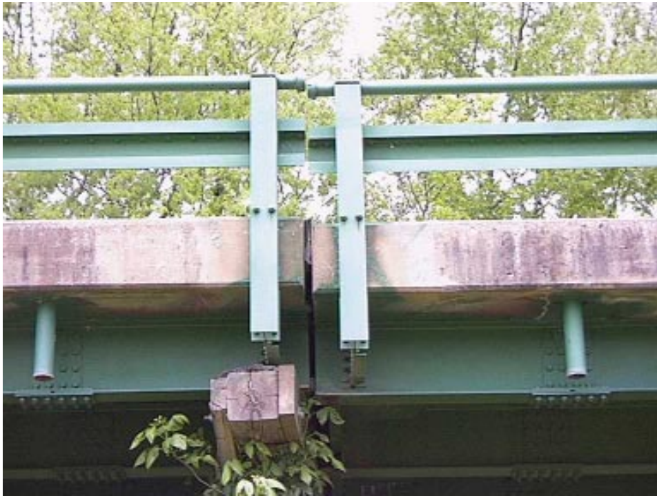
DIFFERENTIAL MOVEMENT OF CURB AND BRIDGE RAILING
