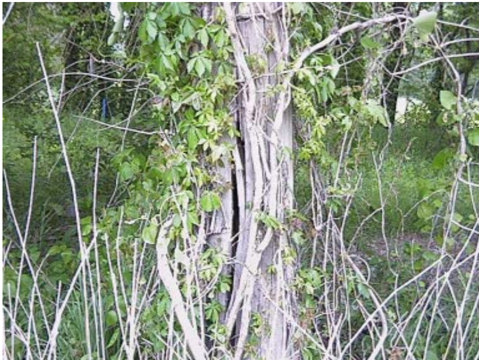
SEVERE DECAY IN EXTERIOR TIMBER PILE "A"
