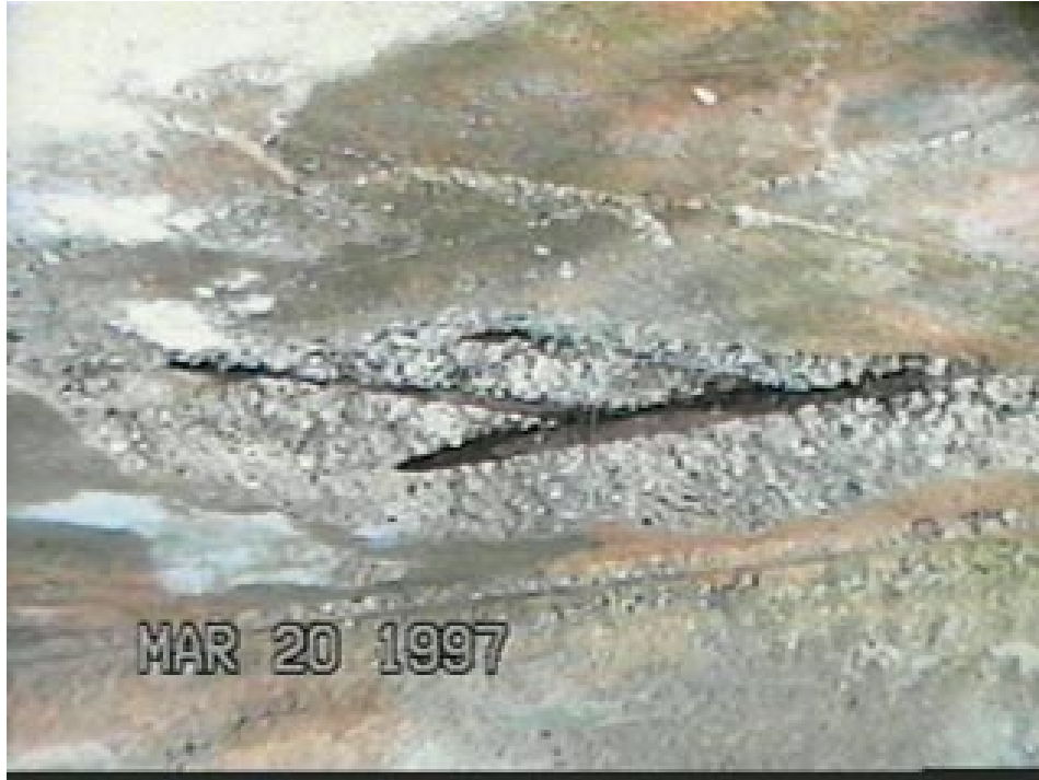
CONCRETE SPALL IN BRIDGE DECK
