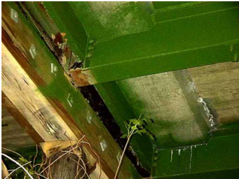
LOSS OF BEARING FOR FIRST INTERIOR BEAM "B"
