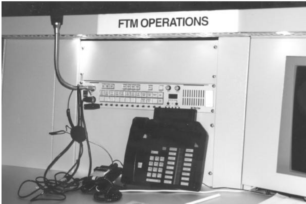
Figure 10-13. Typical Communications Devices Used by Operators in a Control Center.
