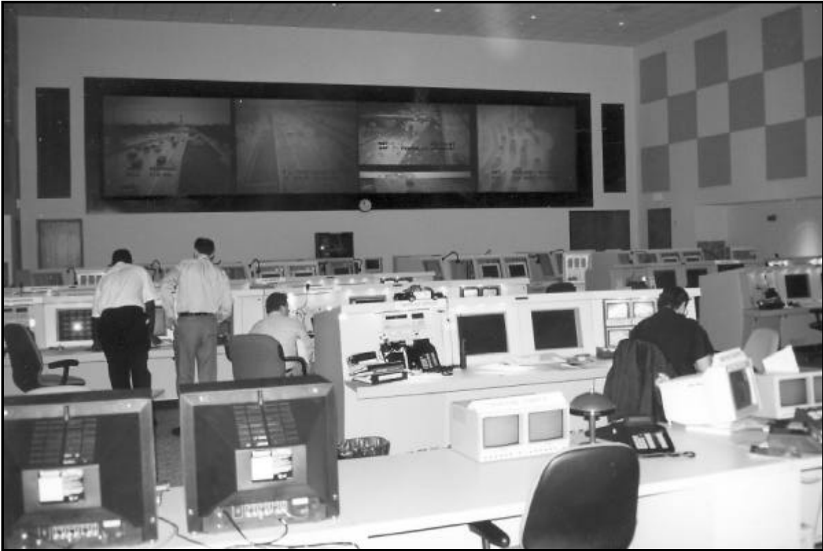
Figure 10-1. The Control Center of the TranStar Freeway Management System in Houston, TX.
