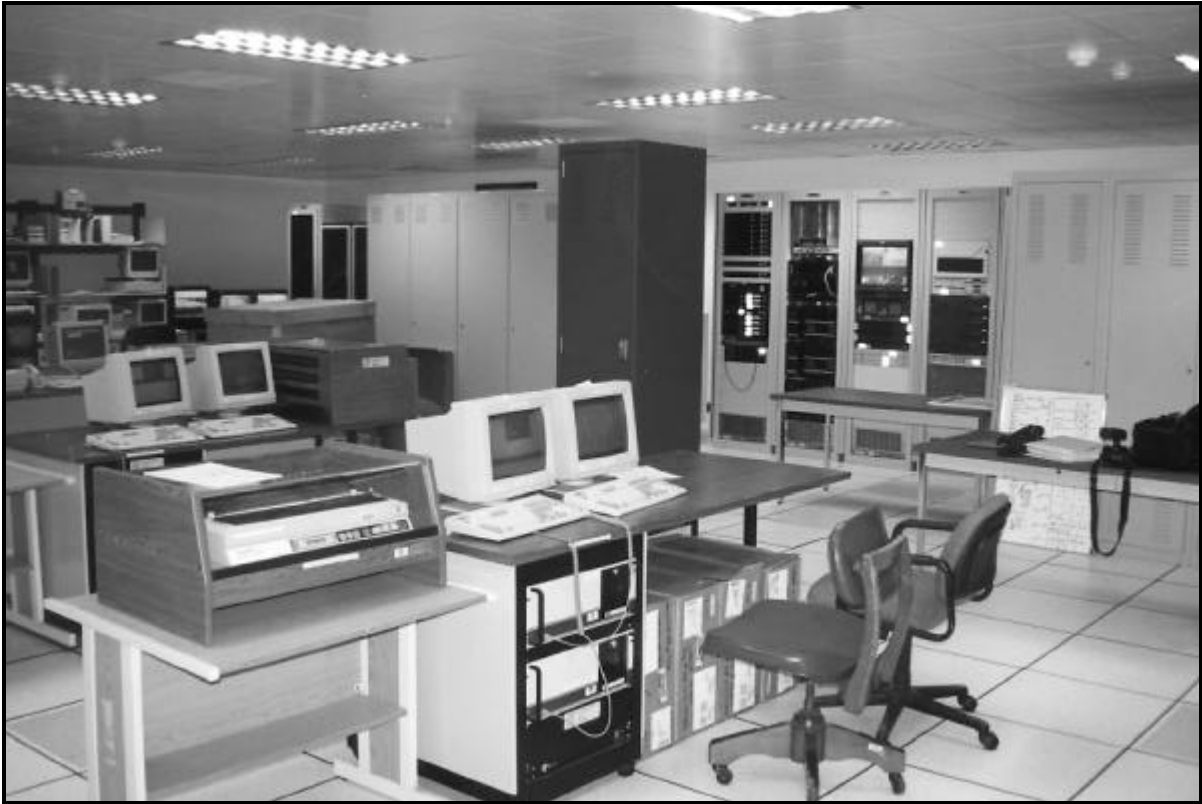
Figure 10-7. Example of a Computer/Peripheral Area in a Control Center.
